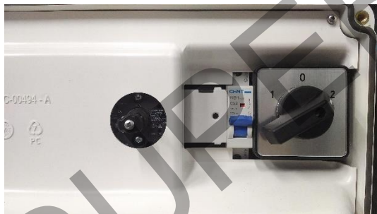
Figure 5: AC Selector Switch in Bypass, inc inner shield
