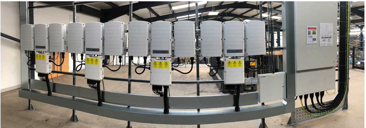
The small footprint and lightweight design of SolarEdge's Three Phase Inverters with Synergy Technology enabled CleanEarth to complete the large-scale installation in just four weeks. It also helped CleanEarth to secure grant funding towards the cost of the project.
