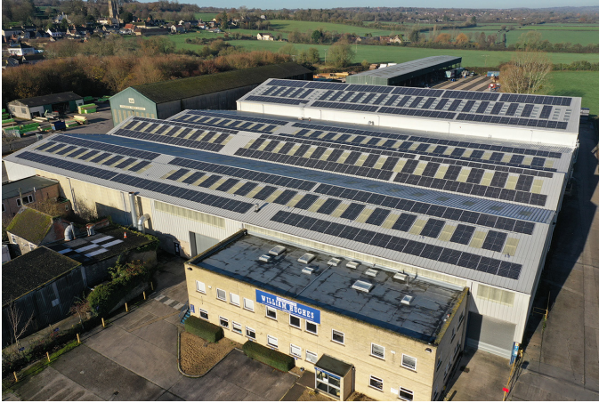
William Hughes expects to cut energy bills by approximately £35,000 and reduce carbon emissions by 100 tons per year using SolarEdge rooftop PV solution.
