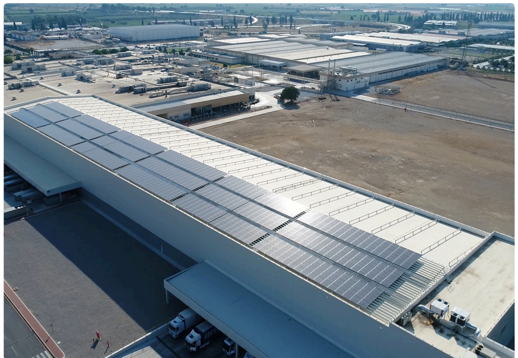
The 514kWp solar PV system was installed on the roof of JTI Torbali's logistics center.
