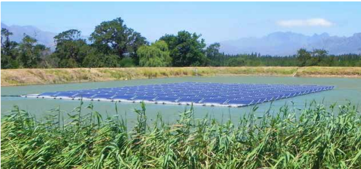
The floating solar system is the first such commercially operational system installed in Sub-Saharan Africa.
