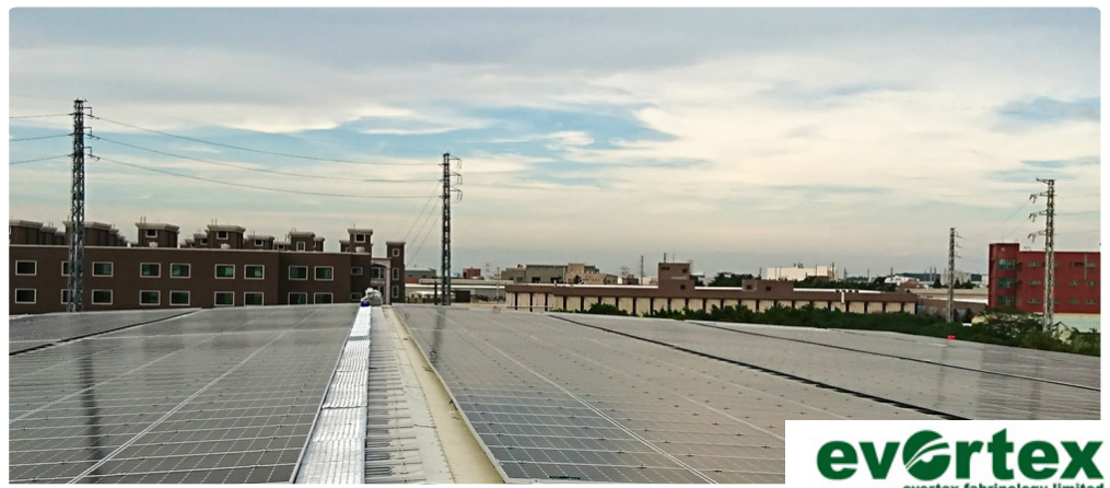
View of PV modules installed on the Evertex factory roof
