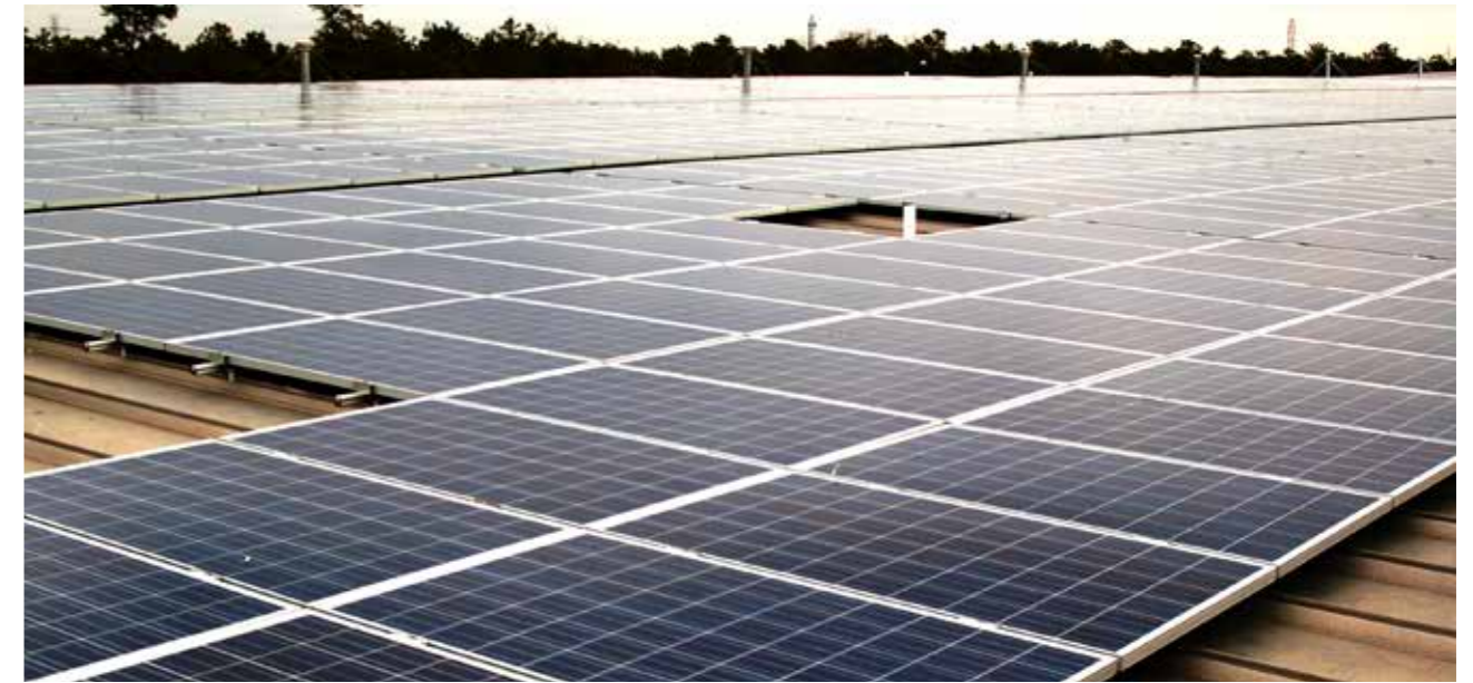
New Jersey, USA, 525 kW
