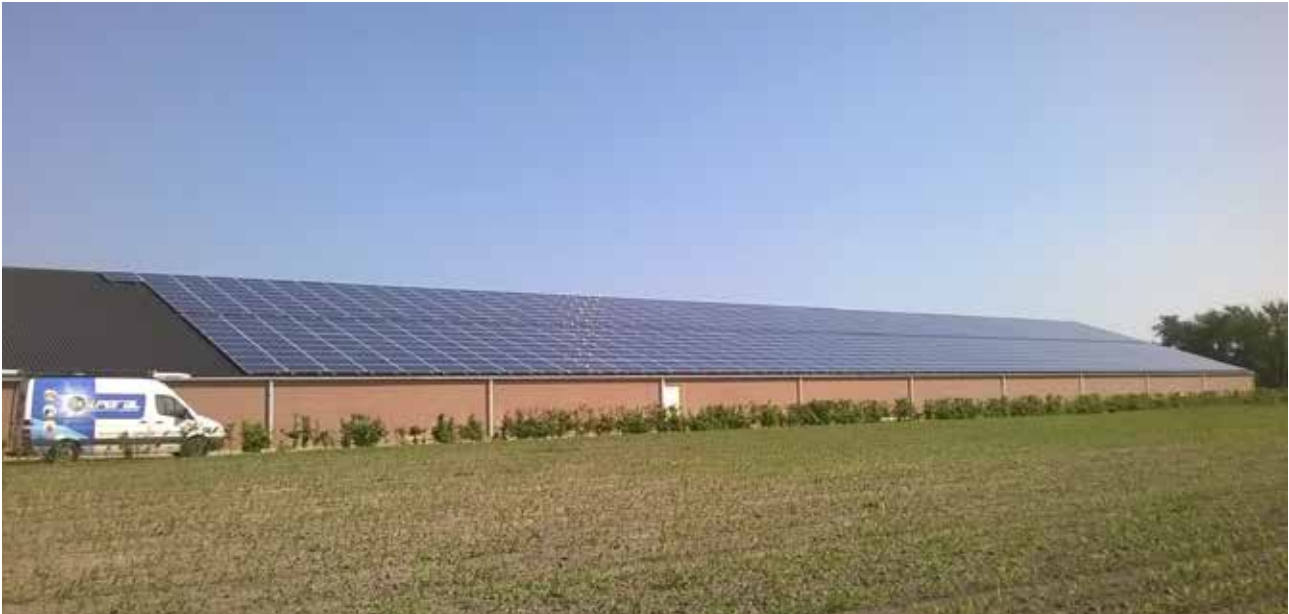
The Netherlands, 303kW
