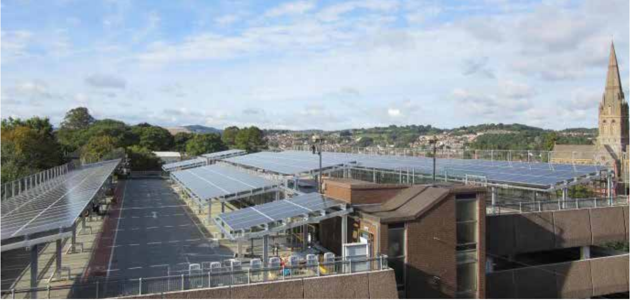
United Kingdom, 150kW John Lewis car park, Exeter
