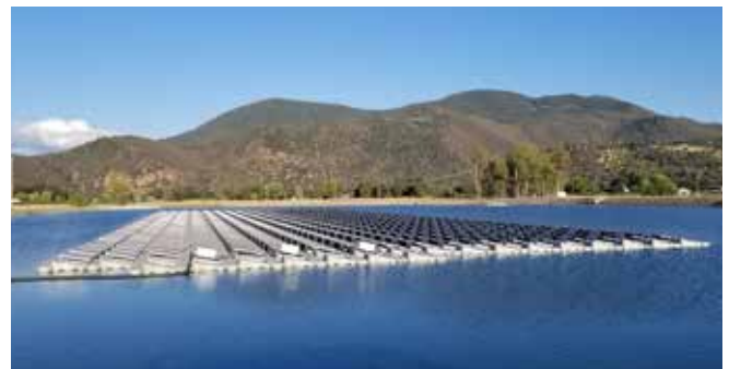
252 kW, Kelseyville Waterworks Floatovoltaic, USA
