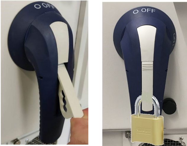
DC ON/OFF switch safety padlock
