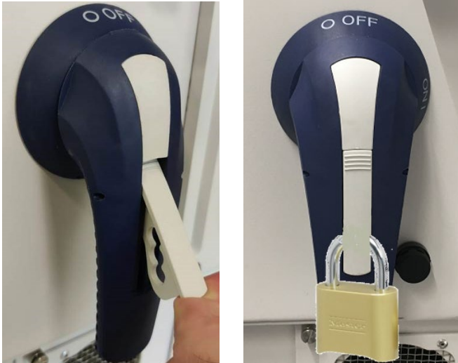
DC ON/OFF switch safety padlock
