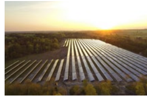
Ground Mount/Community Solar
