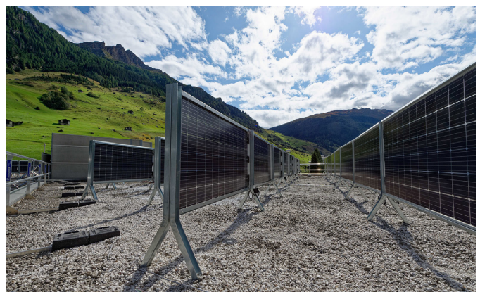
Vertical installation powered by SolarEdge
