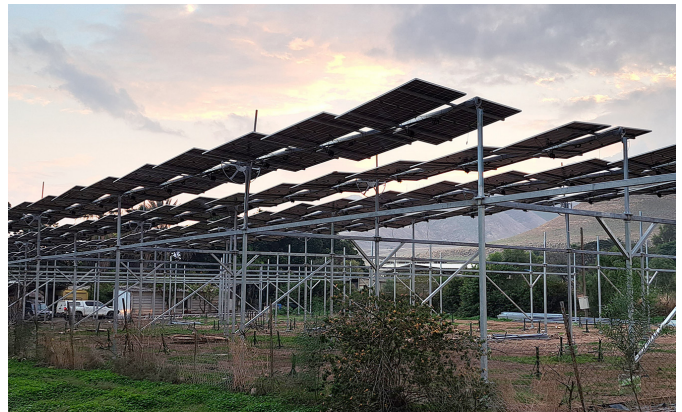
Elevated structure using SolarEdge PV trackers
