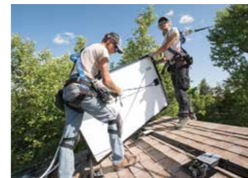
SolarEdge at home
