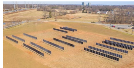
Vertical installation powered by SolarEdge
