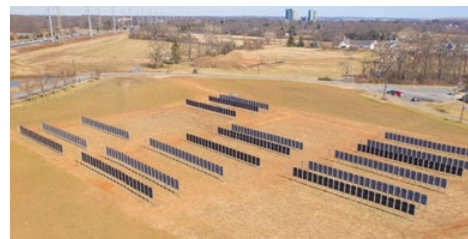
Vertical installation powered by SolarEdge
