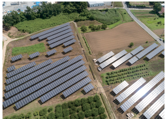
Location: Saitama Prefecture, Japan System Size: 6.705MWdc / 4.861MWac Panel: LONGI Solar 300W x 22,532 panels Solar inverter: SE33.3K-JP x 146 inverters Power Optimizer: P600 x 11,266 power optimizers
